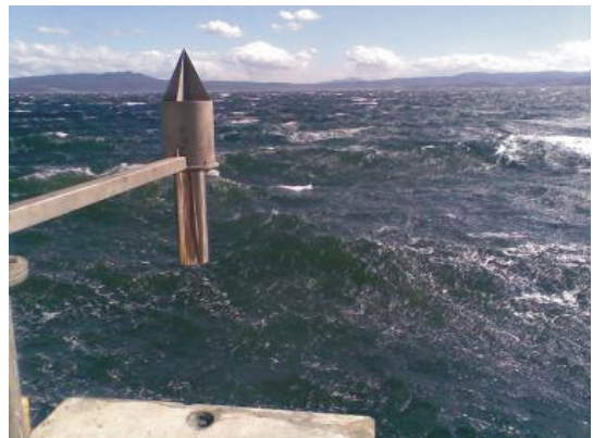
Radar water level monitoring sensor
